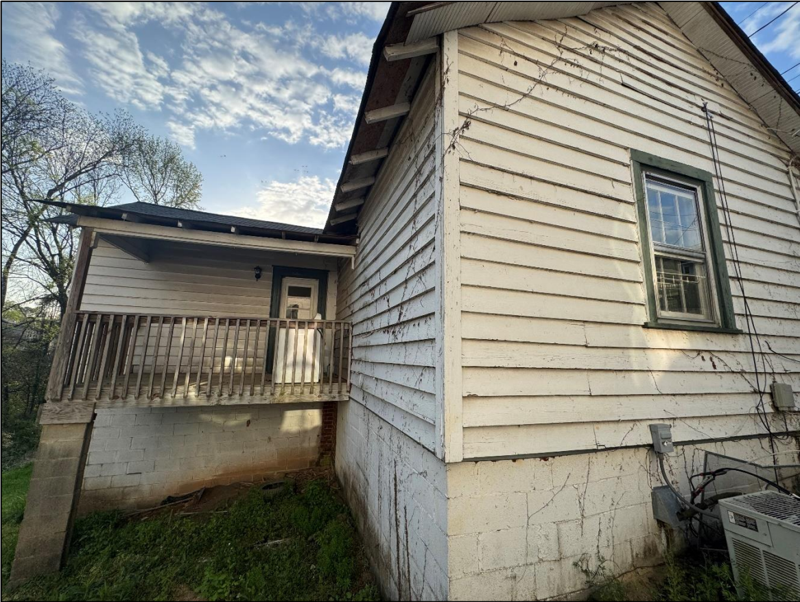
Figure 3. Existing left façade with rear addition and porch visible at 55 Maple Street (photo by Staff)
