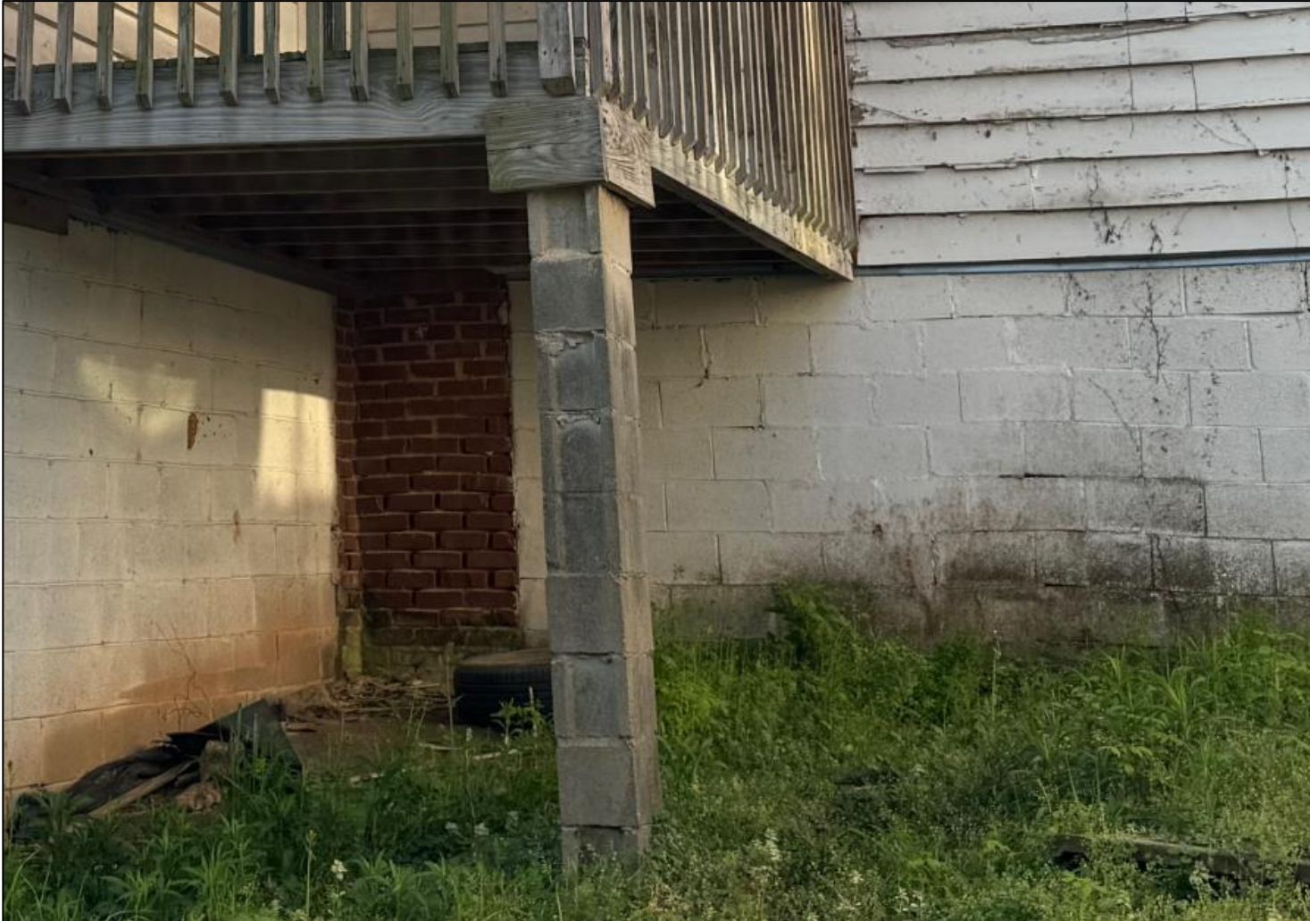
Figure 6. Cinderblock stack holding up rear porch; water damage on cinderblock wall also visible in exterior Staff observations (photo from Staff)
